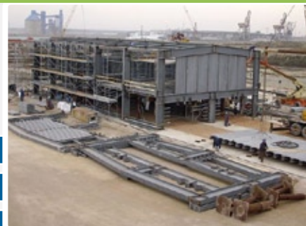
Installazione Mouli Local Equipment Room per Agip KCO Kazakhstan Kazakhstan - Mouli Local Equipment Room installation
