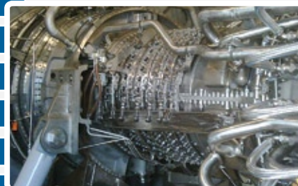
Marghera LMS100 ( turbine a gas) Marghera - Gas turbine installations LMS100
